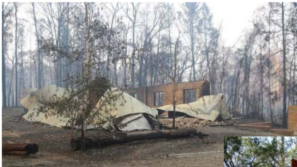
Above: SouthWest view of the destroyed Kitchen / Dining room
